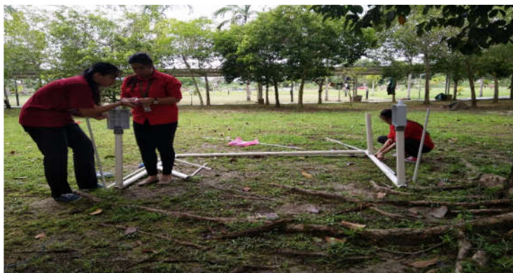
Figure 5: Proseses of Configuring Each station with the Passive Devices and Fiber Optics Cable
